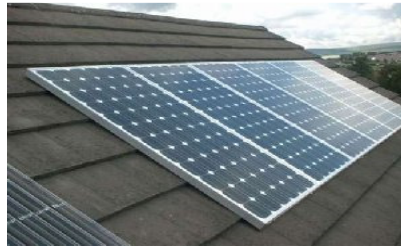
Figure 1 - Roof Mounted Photovoltaic (PV) Panels
